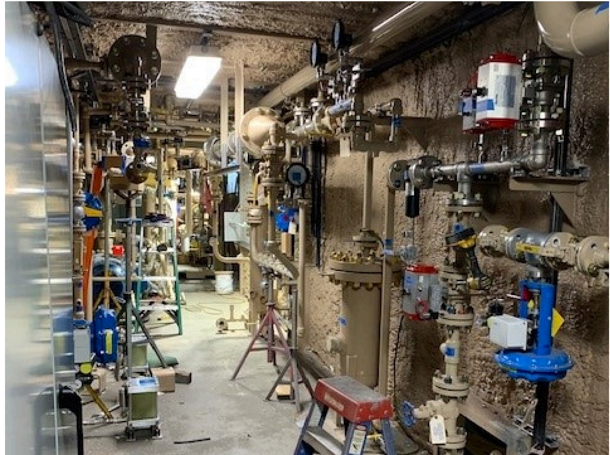
Internal view of 1 of the 4 modular housing units that house the helium processing facility
